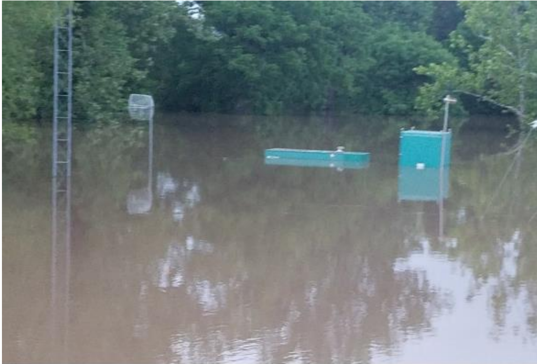
Pump Station 20: Photo taken May 28, 2019
