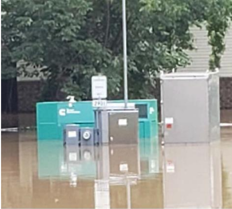
Pump Station 21: Photo taken May 28, 2019
