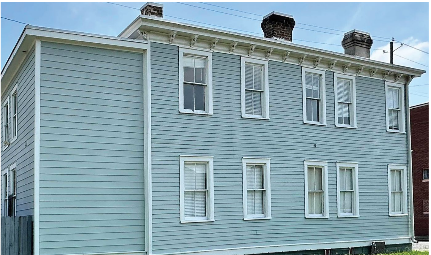
Figure 7. A new addition replaced non-historic construction on the rear elevation of this building. Fiber cement gives the addition a compatible appearance without replicating the exposure for thickness of the historic siding. Photo: Ward Architecture + Preservation.
