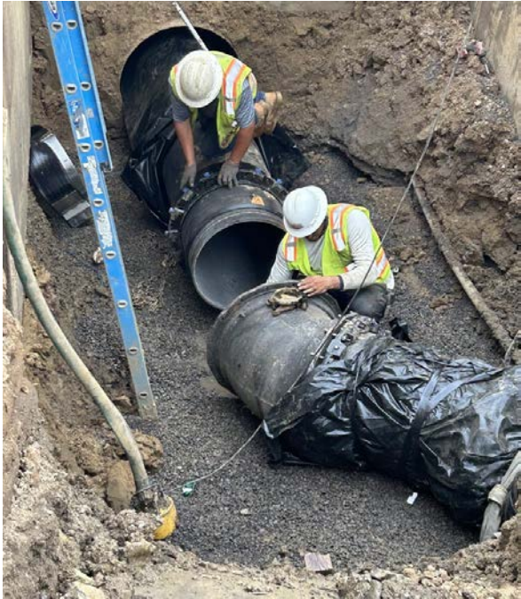
24-Inch Water Transmission Pipe Fitting
