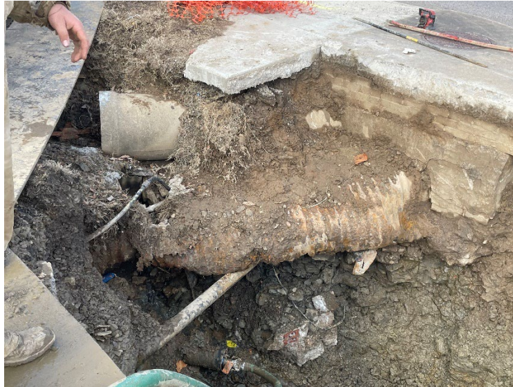
Line 8 – Deteriorated Storm Water Culvert Next To Manhole
