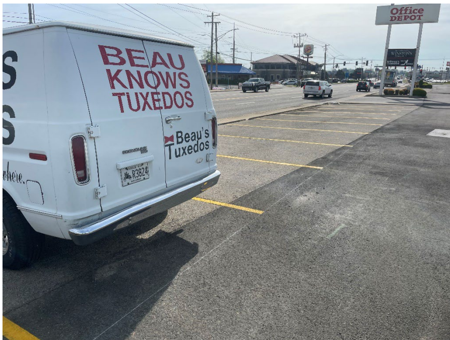
Line 8 – Asphalt Patch
