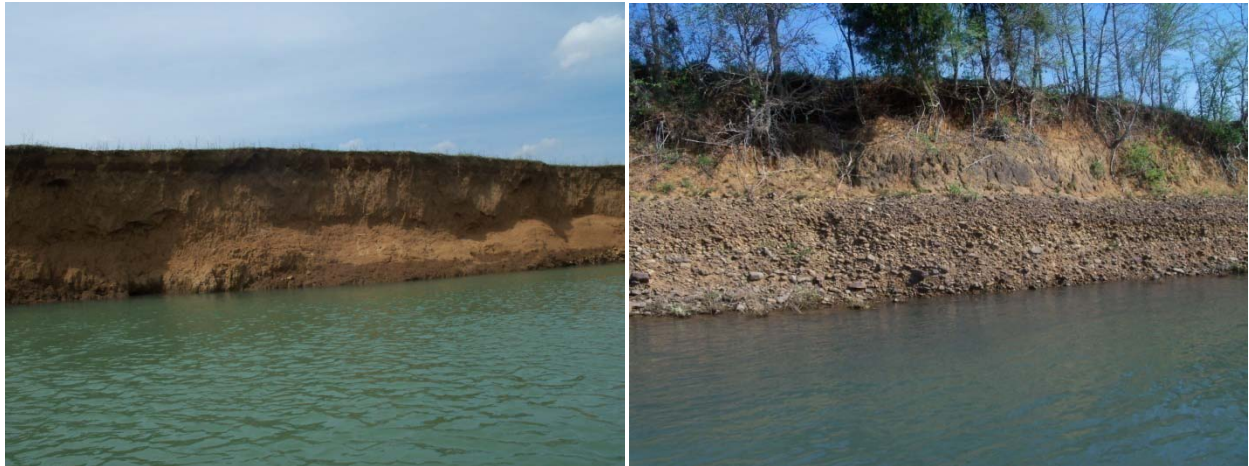
Figure 17. Stream Banks with Very High Bank Erosion Hazard in Lower Lee Creek.
