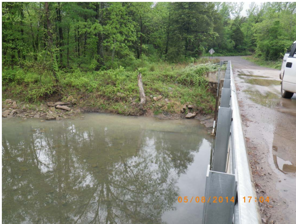
Figure 24. Sediment Plume entering Cove Creek from Unpaved Road Runoff.
