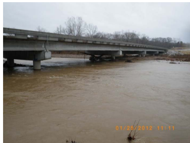
Figure 12. LLC-2 during Storm Event.
