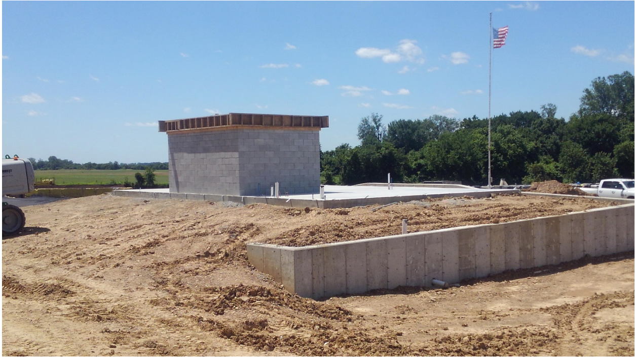
LWCMU wall complete at Copy / File Room at Office / Scale House. Note underfloor plumbing completed as well as concrete slab.
