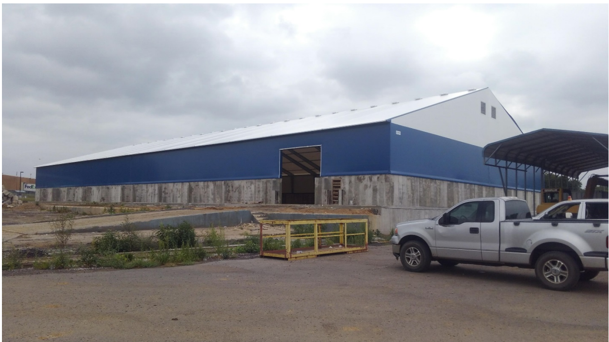
Warehouse 1 – West Side. Building is nearing completion with the exception of exterior doors and electrical power.
