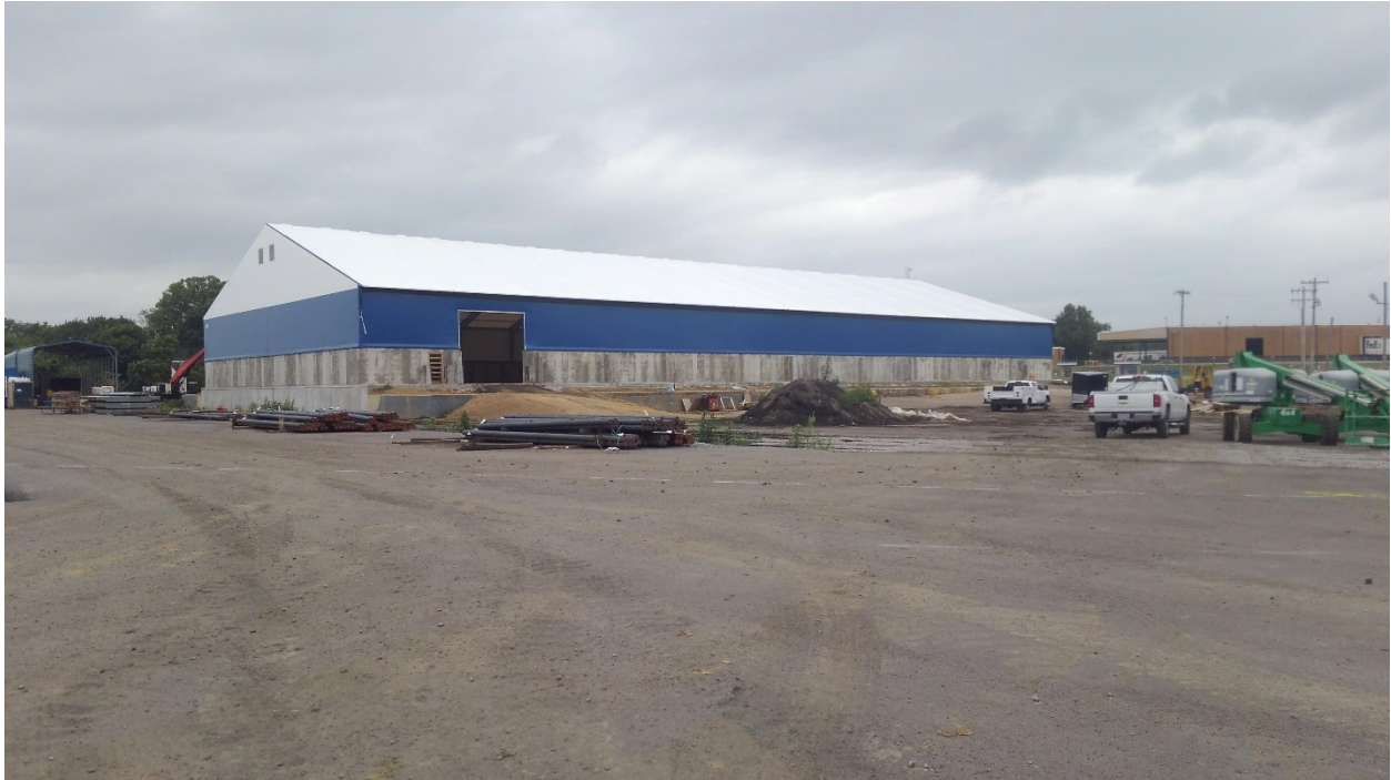
Warehouse 1 – East Side. Building is nearing completion with the exception of exterior doors and electrical power.
