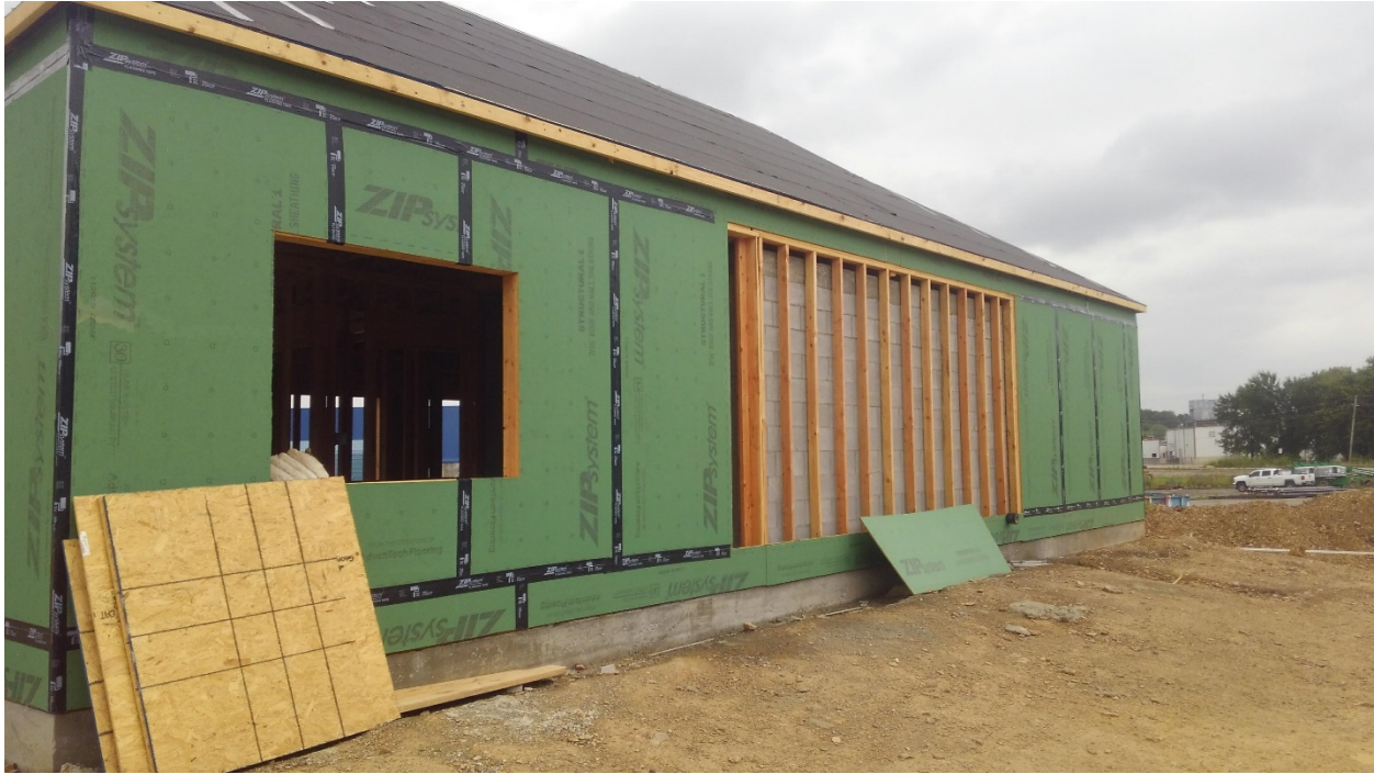
Scale House / Office. Building is framed and sheathed with the exception of the exterior wall sheathing at the Copy Room awaiting exterior wall insulation.
