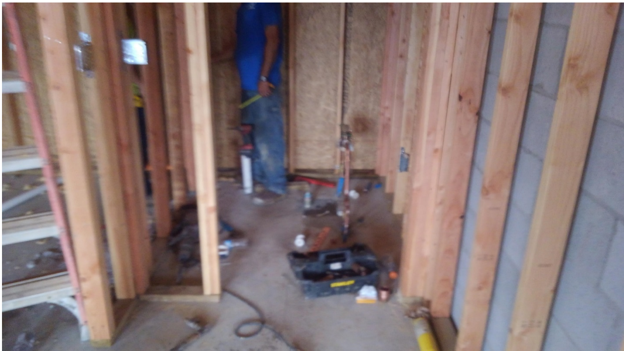
Plumbing RPZ installed in Janitor – 103 at Scale House / Office.
