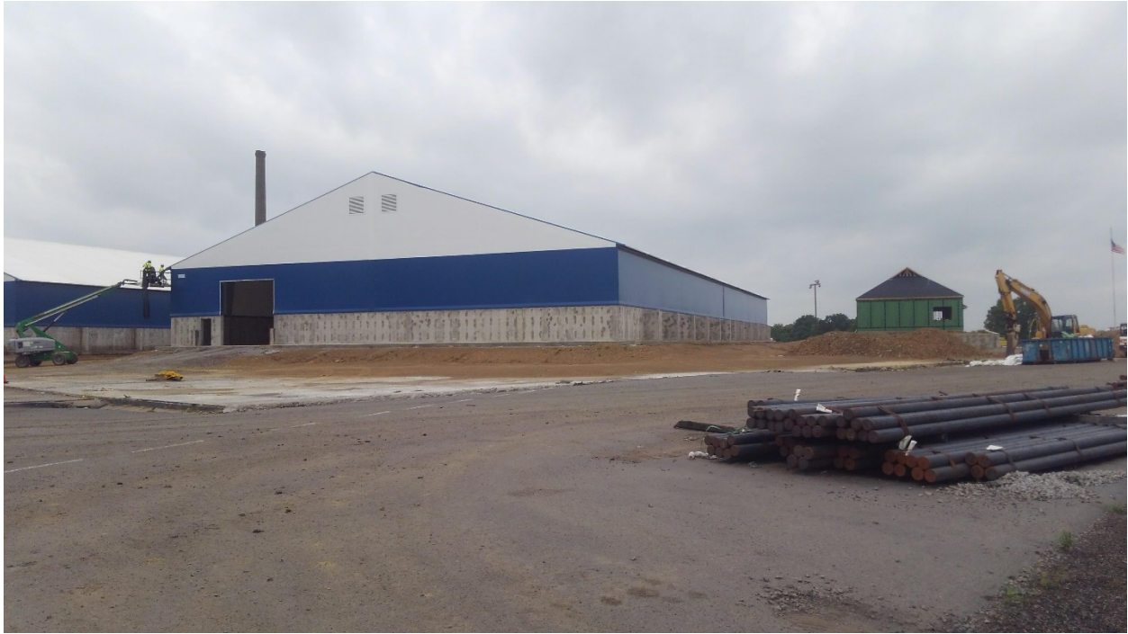
Warehouse 2 – East End. Building is nearing completion with the exception of exterior doors and electrical power.
