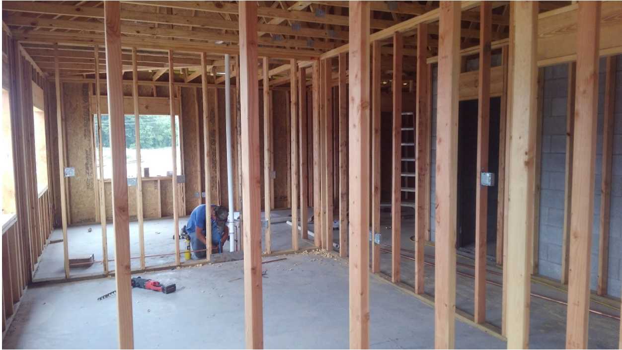
Interior framing at Scale House / Office. Note Plumbing Contractor installing plumbing supply lines at Break Room – 107.
