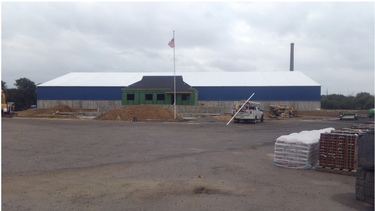
Warehouse 2 – North Side. Building is nearing completion with the exception of exterior doors and electrical power. Note Scale House / Office in foreground.
