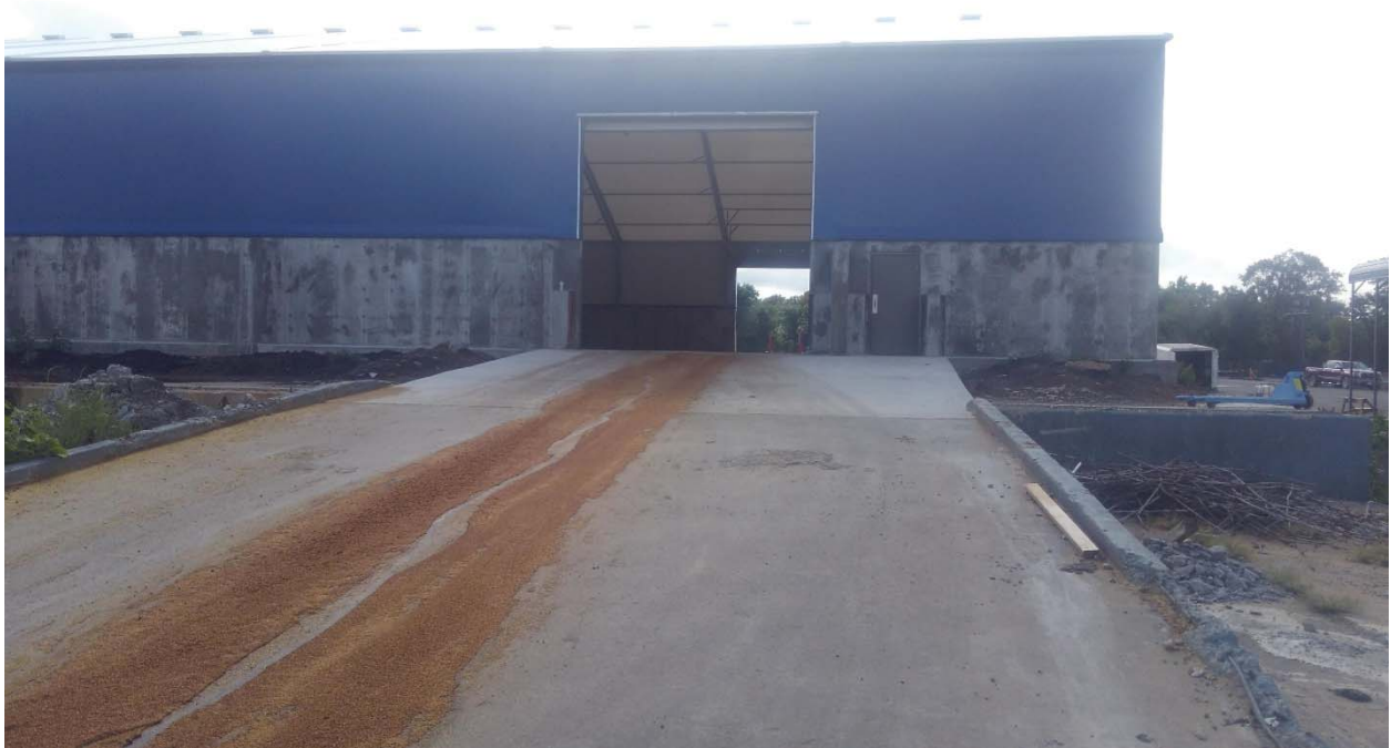
Concrete Ramp completed on North side of Warehouse 1. The City has issued a Temporary Certificate of Occupancy for Warehouse 1 and Operator is currently using building.
