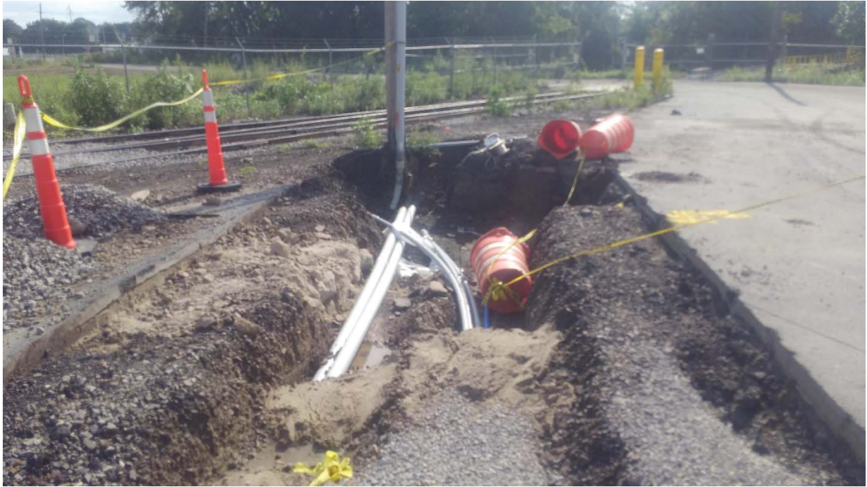
Electrical conduits have been installed from Transformer Pole to Scale House / Office as well as from Scale House / Office to Small Dock. OG&E is working on scheduling electrical tie-in to system.
