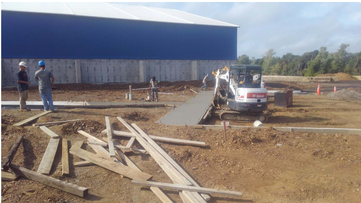
Concrete sidewalk / curb at Parking Area on the West side of the Scale House / Office being completed this date.
