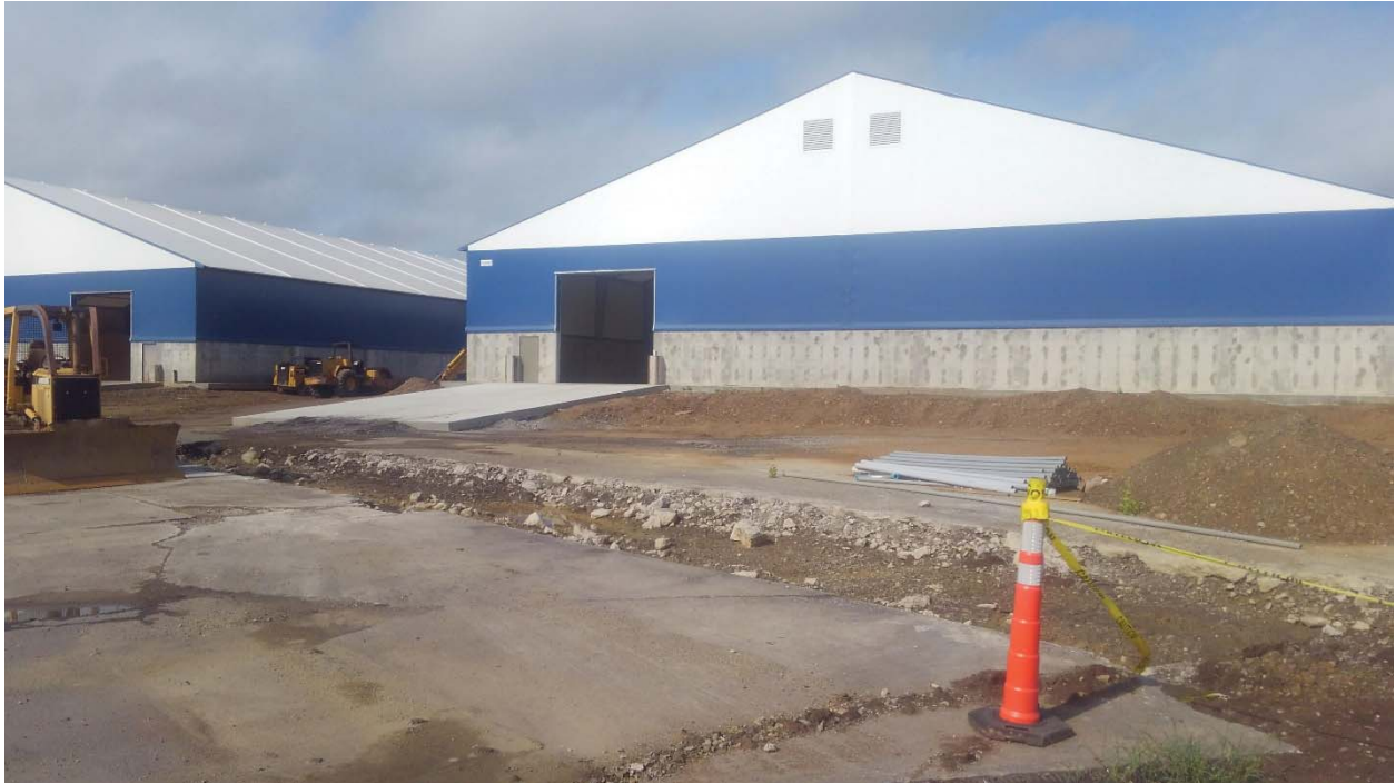
Concrete Ramp completed at East end of Warehouse 2 with dirt work being completed for gravel pavement tie-in.
