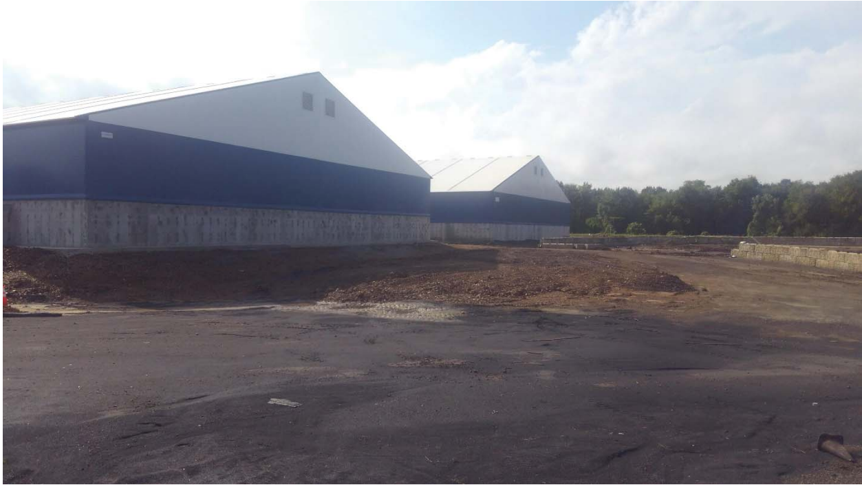
Dirt work continuing on the West and South sides of Warehouse 2 in preparation for pavement installations.
