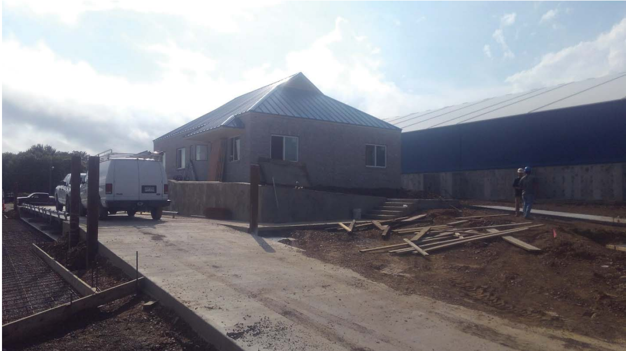
Exterior work at Scale House / Office is nearing completion. Roof has now been installed as well as perimeter sidewalks / steps.
