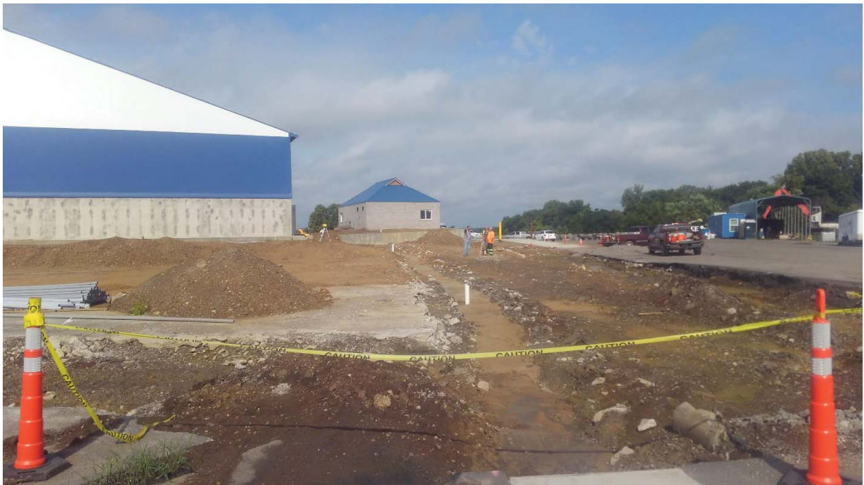
Dirt work continuing on the North and East sides of Warehouse 2 in preparation for pavement installations.
