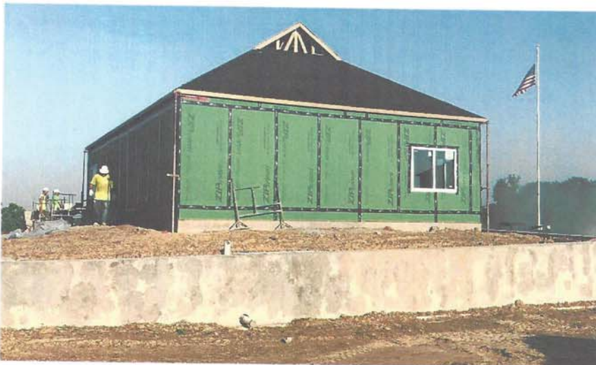
Photo Two Caption South side of building facing North along the South side and back of building.
