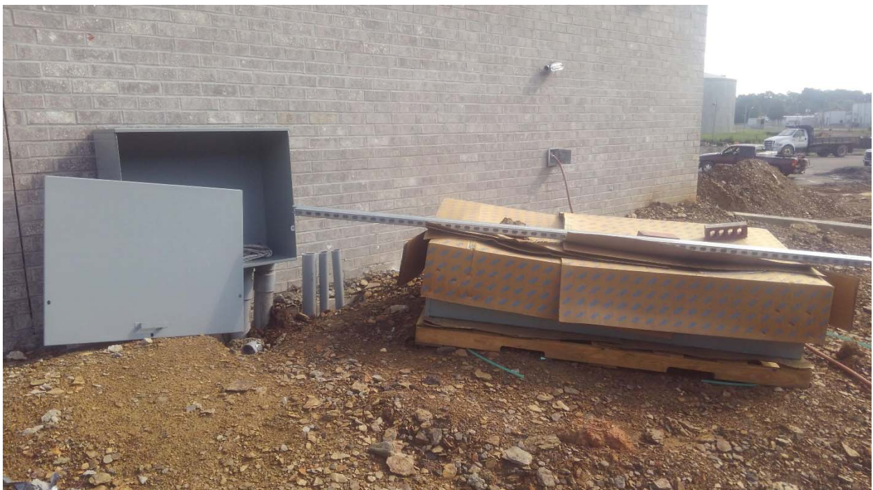
Electrical MDP at Scale House / Office installed with electrical conduits to Transformer Pole.
