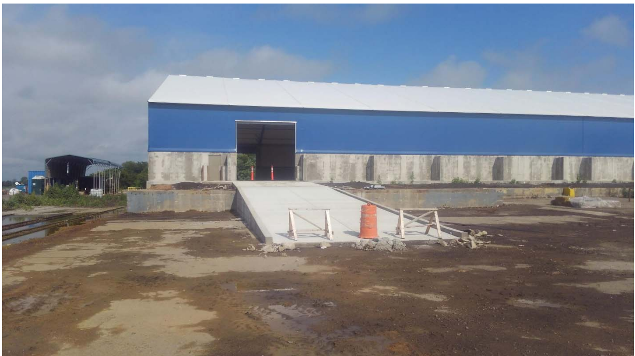
Concrete Ramp completed on South side of Warehouse 1. The City has issued a Temporary Certificate of Occupancy for Warehouse 1 and Operator is currently using building.
