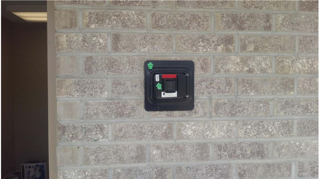
“Knox Box” as required by the City of Fort Smith Fire Department has been installed at the Scale House / Office main entry.
