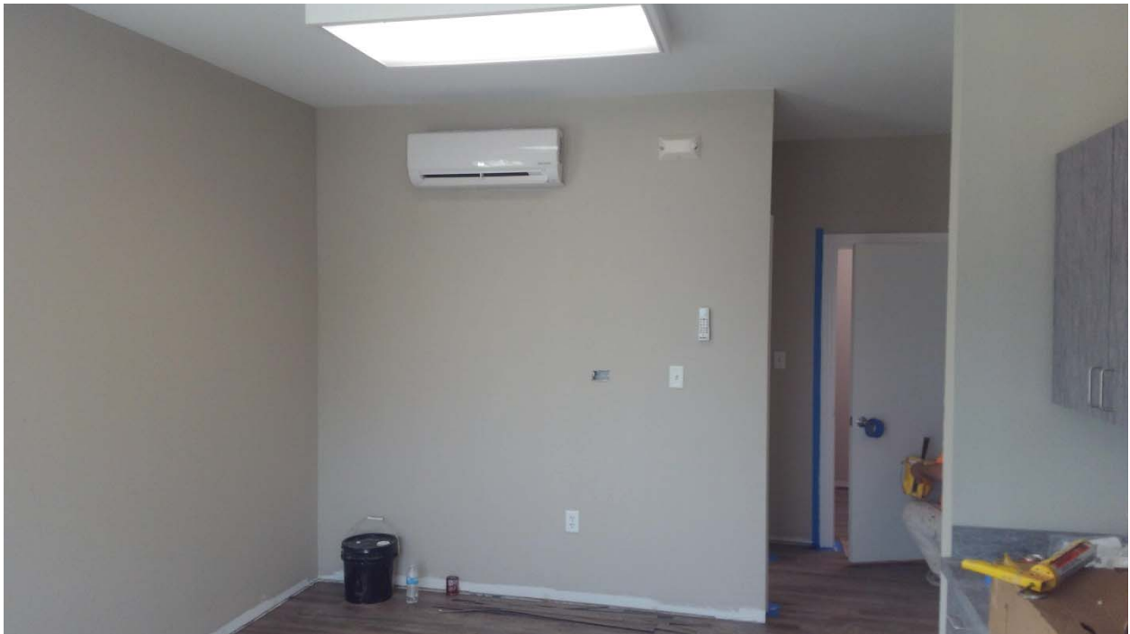
Indoor HVAC Unit installed in Break Room at Scale House / Office.
