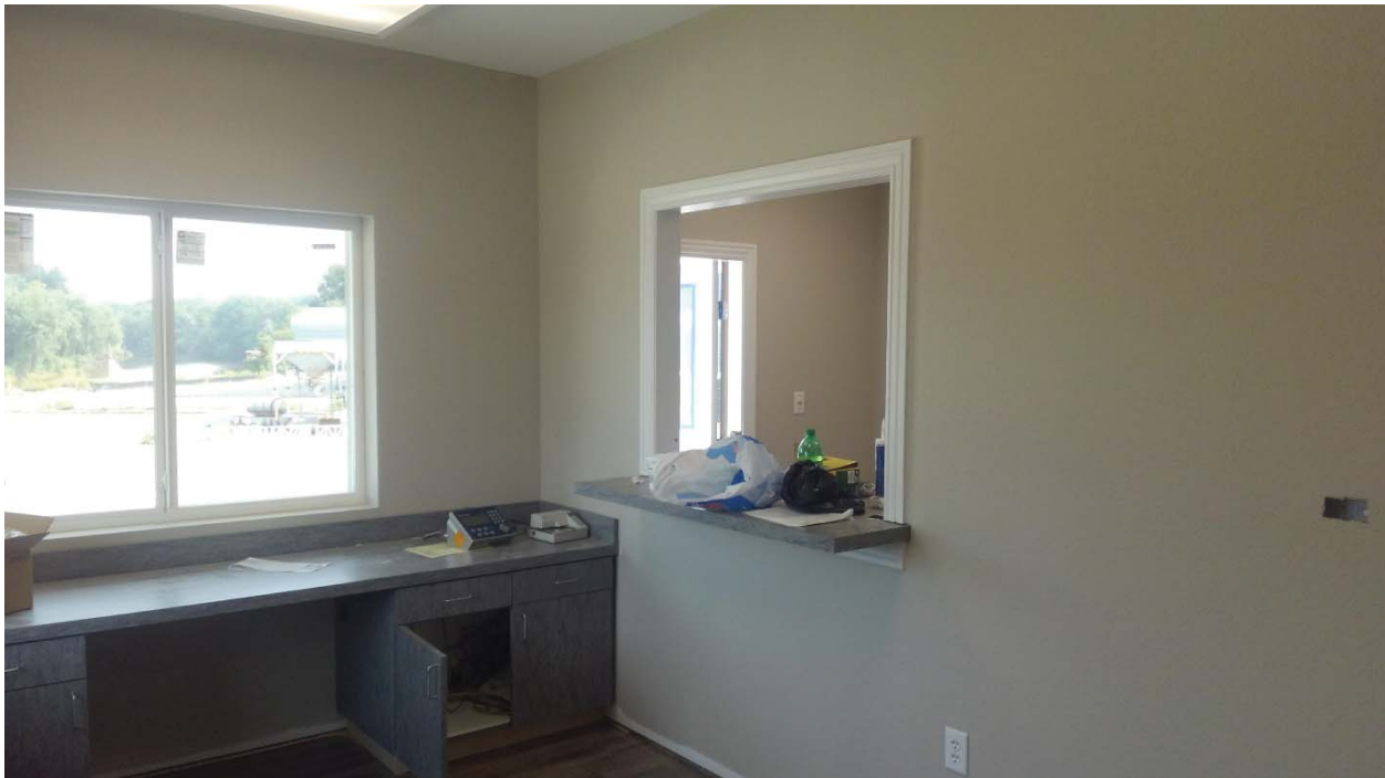
Millwork installation, including deal window and counter at Scale Office in Scale House / Office.
