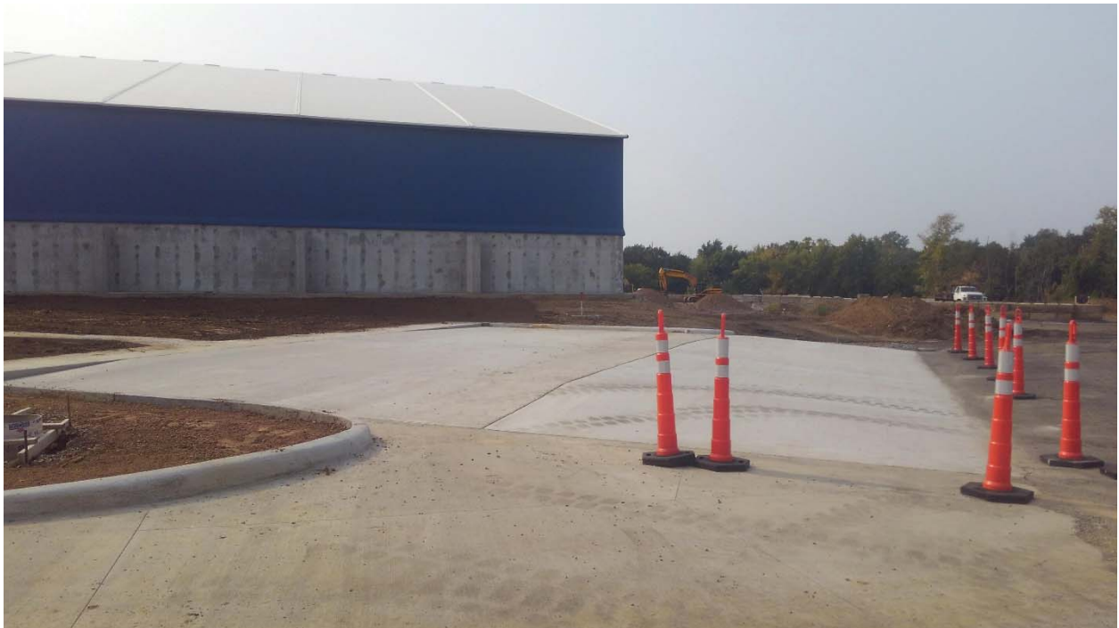
Parking lot pavement completed (with exception of painted stripes) on the West side of Scale House / Office.
