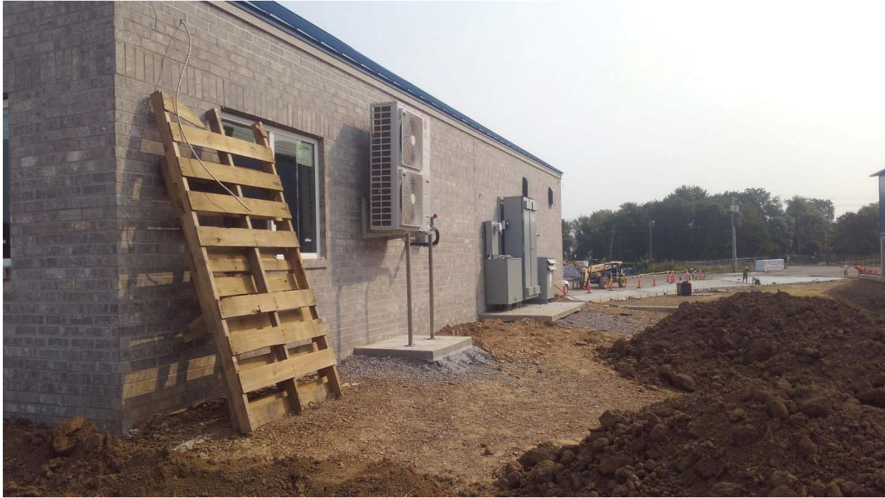
Outdoor HVAC Units installed on the South exterior wall of Scale House / Office.
