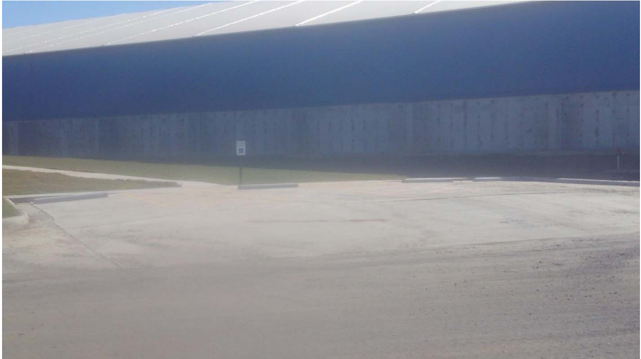
Painted parking stripes have been completed at the Parking Area on the West side of the Scale House / Office.
