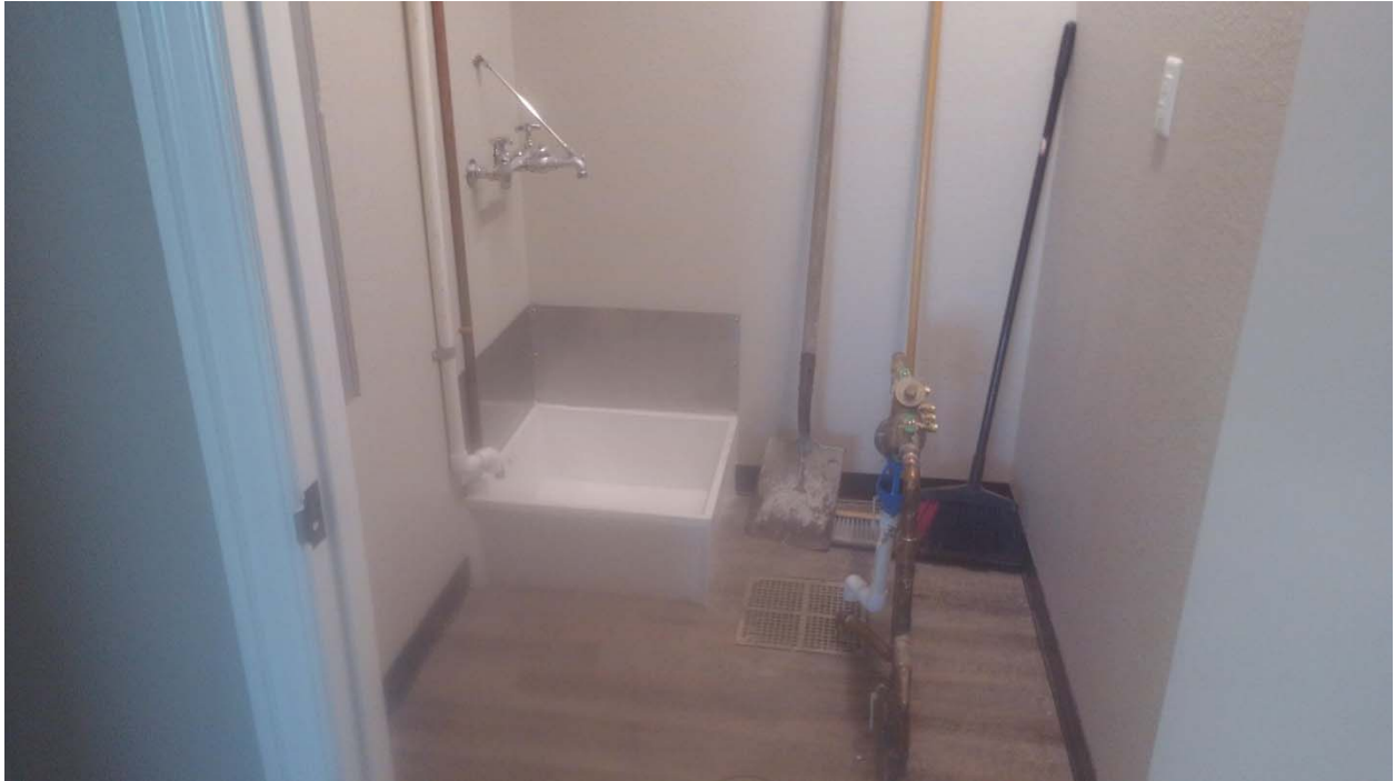
Plumbing top-out has been completed in the Janitor Closet of the Scale House / Office.
