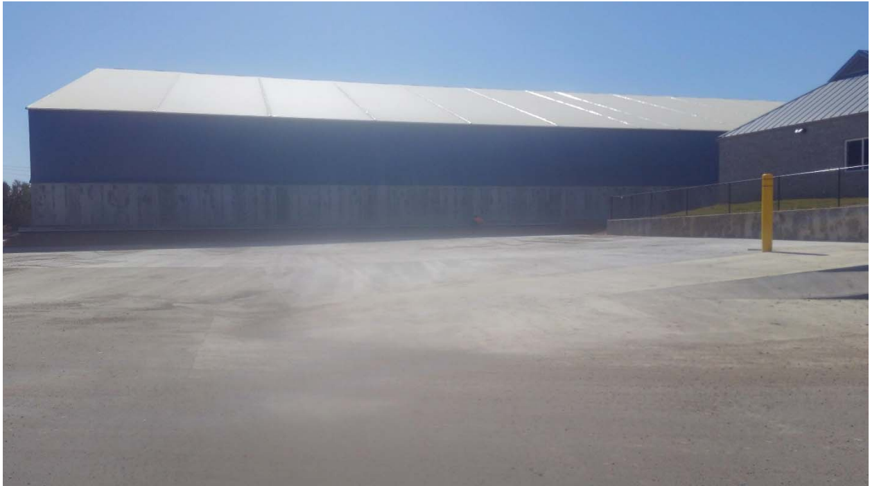
Site pavement completed on the North side of Warehouse 2 with the exception of the sloped strip between flatwork and Warehouse 2 foundation. Area is being prepared for pavement.
