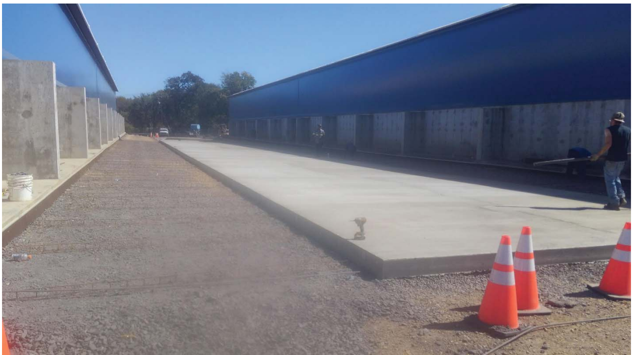
Approximately 25% of the site pavement between Warehouse 2 and existing Warehouse 3 has been completed. Reinforcing is being placed for balance of concrete to be completed within the next 10 days.
