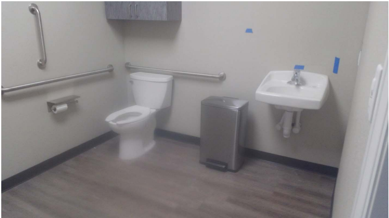
Plumbing top-out has been completed in the Bathroom of the Scale House / Office.
