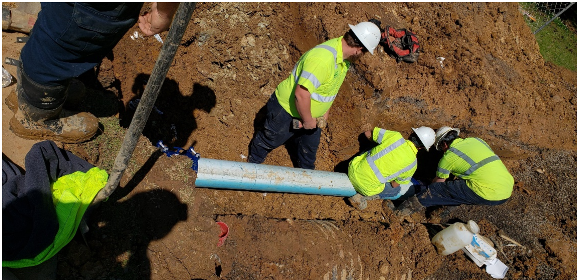
Fort Smith Utility Crew works to replace a broken water line over Easter Weekend 2020
