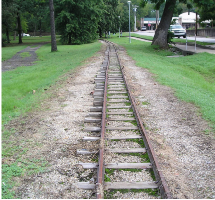
Example of railroad tie issue.
